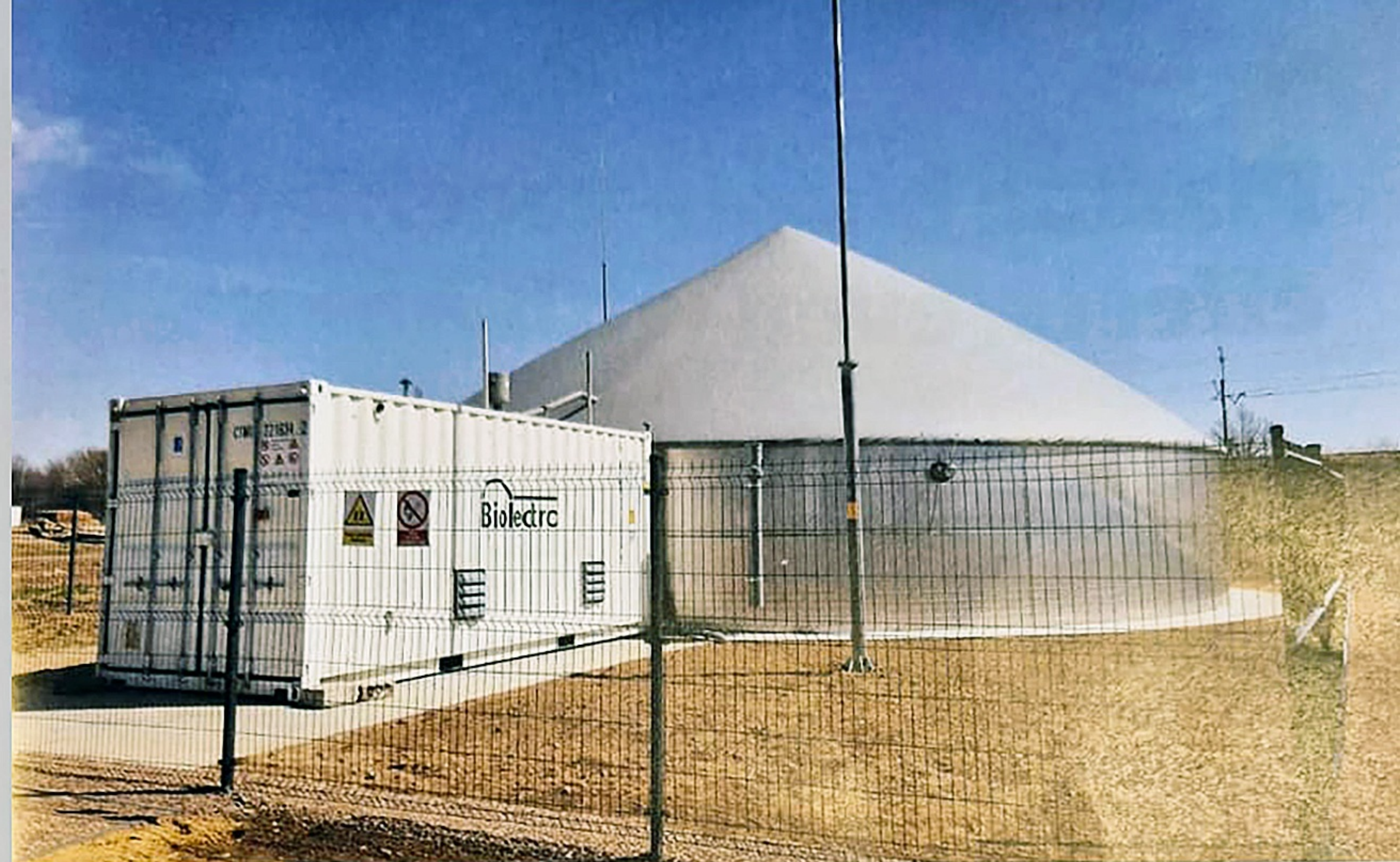
A mini-biodigester as supplied by Bioelectric.
